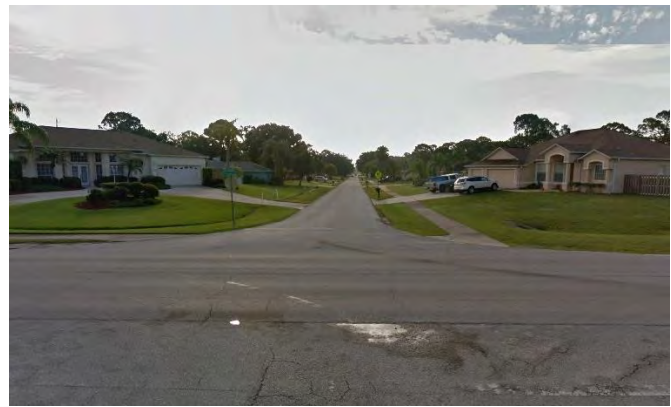
Sidewalk Gap At Narragansett Street
