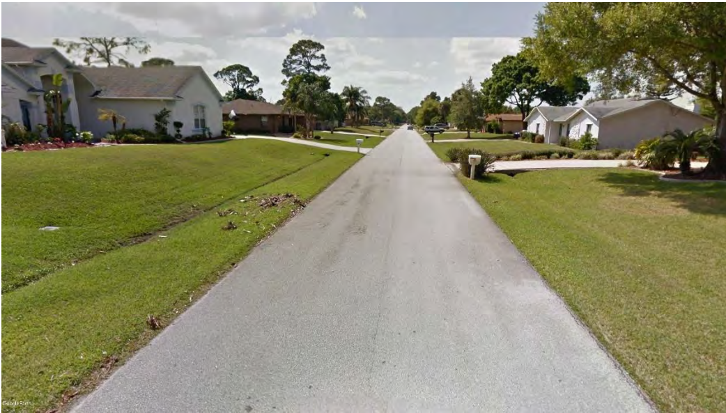
Sidewalk Gap Along Narragansett Street
