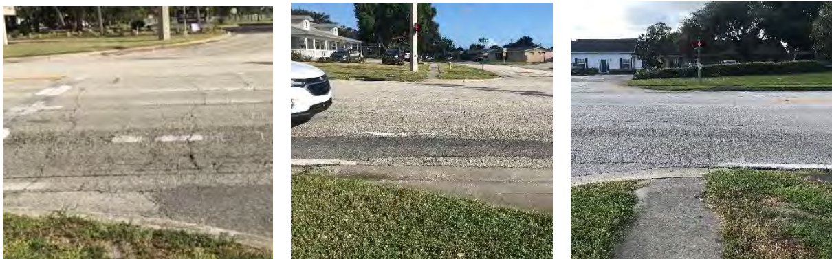
No Pedestrian Ramps and Faded Crosswalks Along Sarno Road
