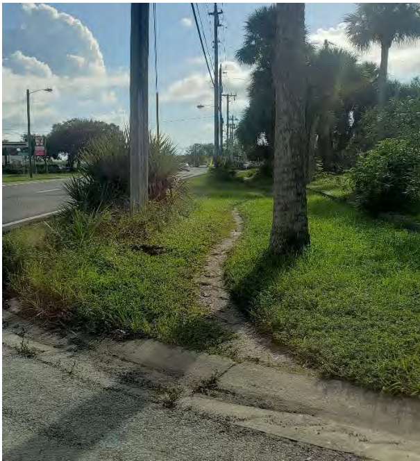
Existing Sidewalk Gap
