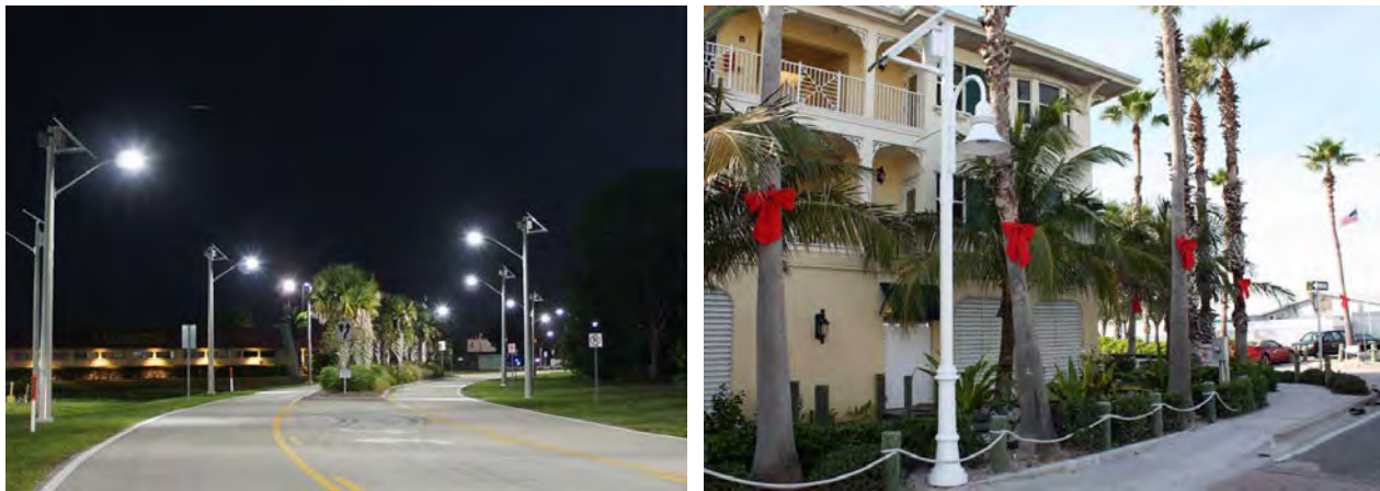
Figure 44: Solar Power Lighting Alternatives
