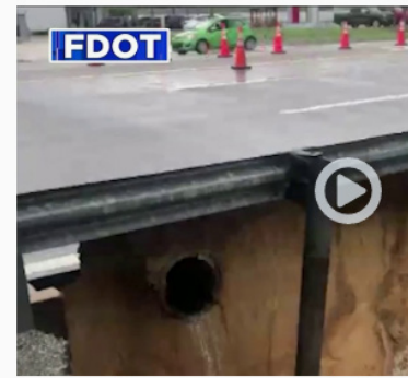
Erosion on the banks of the Indian River due to recent heavy rains and flooding has prompted northbound lanes on a stretch of U.S. Highway 1 in Melbourne, according to city officials.
